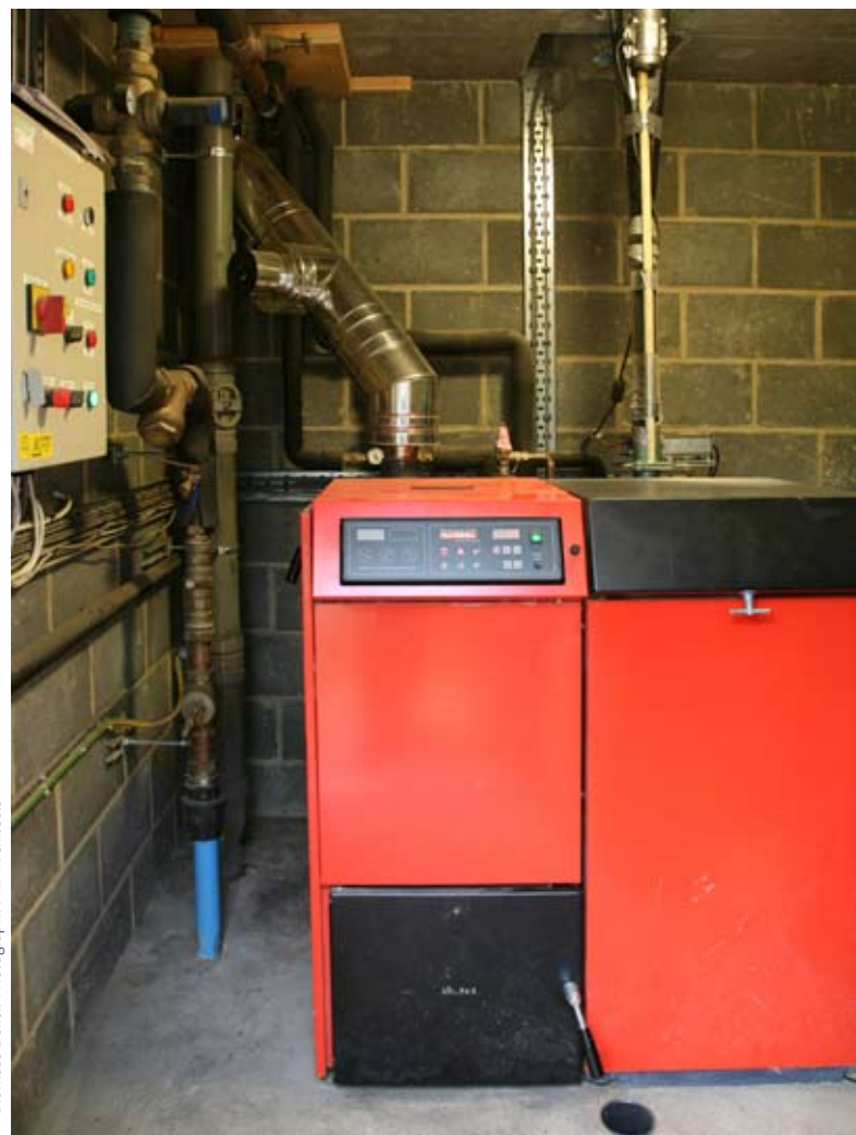
Biomass Boiler. Photograph: PRP Architects
